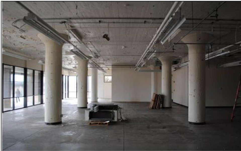
Figure 16. Interior view of Building 18, in southeast corner lobby, looking south; concrete mushroom columns and concrete ceiling are historic and many like this can also be seen below in Figure 46, below. Tallgrass Archaeology LLC photograph, 2/28/2025.
