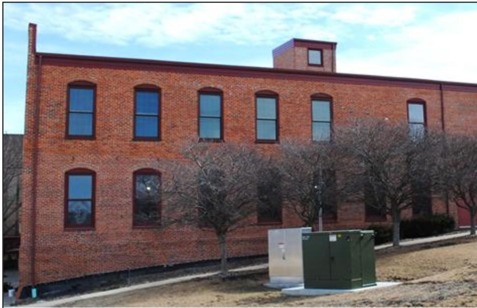
Figure 10. North part of Building 2's west wall, looking east. Notice the difference in color from the historic bricks to those used during the reconstruction of that section after the 2020 derecho. Tallgrass Archaeology LLC photograph, 2/28/2025.
