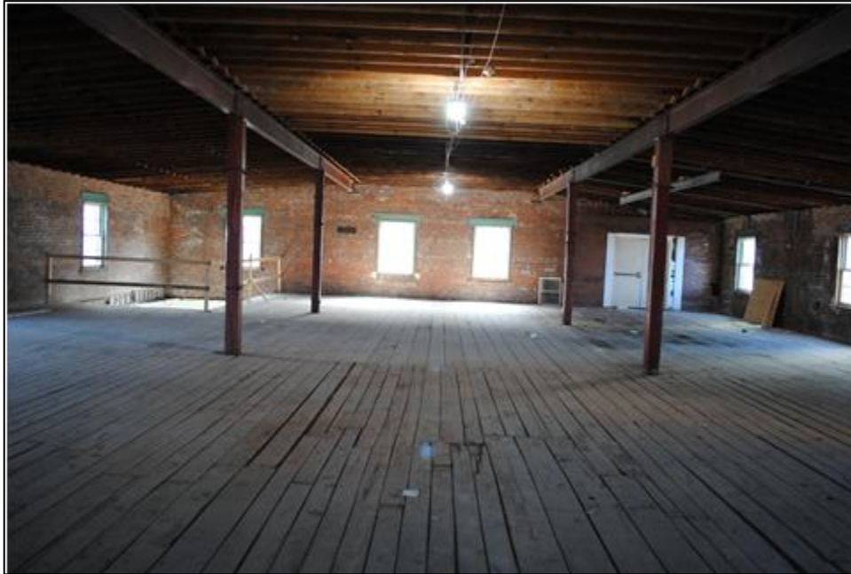
Figure 6. Interior view on top story of Building 1, looking south. Tallgrass Archaeology LLC photograph, 2/28/2025.
