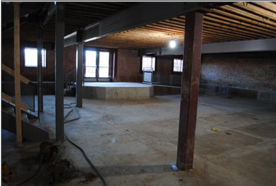
Figure 7. Interior view of lowest level of Building 1, looking northeast. Note the addition of the poured concrete landing inside the doorway and the concrete ramp to the right. Tallgrass Archaeology LLC photograph, 2/28/2025.
