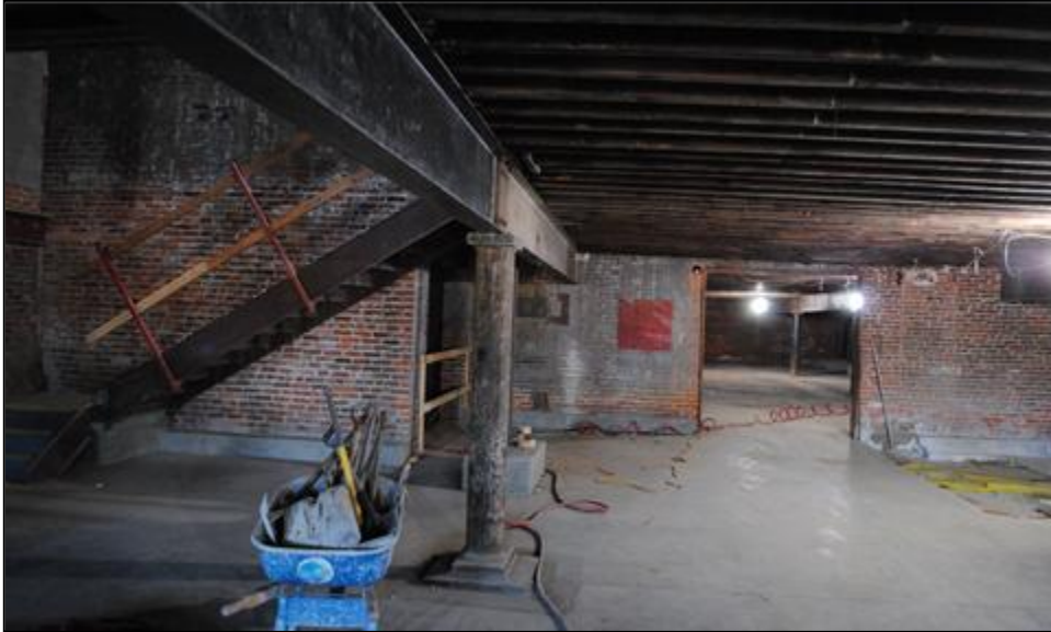
Figure 8. Interior view of Building 2 first story, looking south. Tallgrass Archaeology LLC photograph, 2/28/2025.
