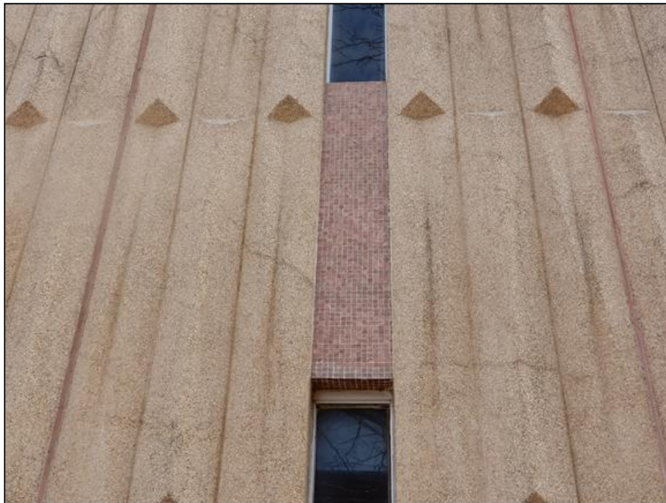
Figure 19. Detail view of aggregate concrete exterior material, tile covering between windows and aluminum windows on west wall of Building 20, looking east. Tallgrass Archaeology LLC photograph, 2/28/2025.
