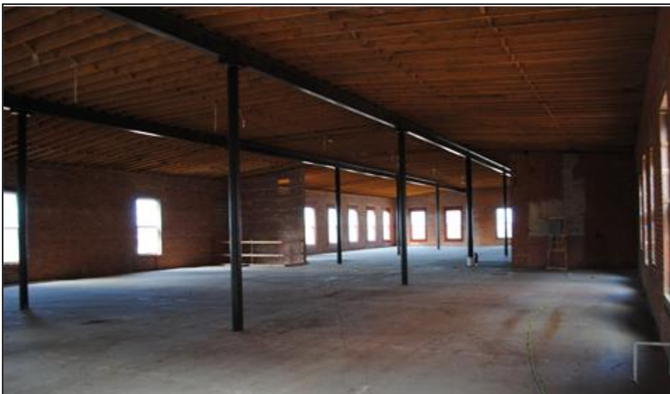
Figure 9. Interior view of Building 2 second story, looking northwest. Tallgrass Archaeology LLC photograph, 2/28/2025.
