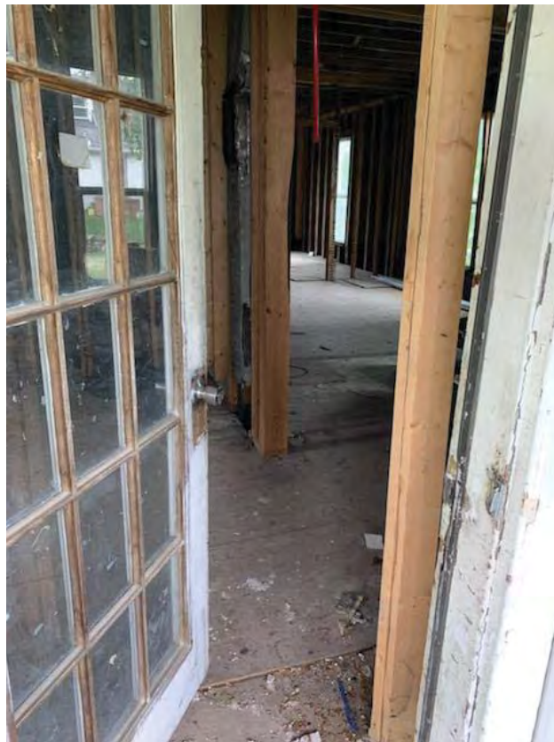
Above: The front and rear of the home. Below: Unsecured rear door. City Nuisance Program has recently mowed the property.
